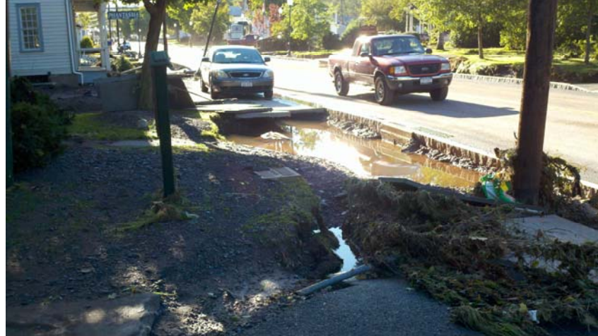
Damage to right driveway and sidewalk
