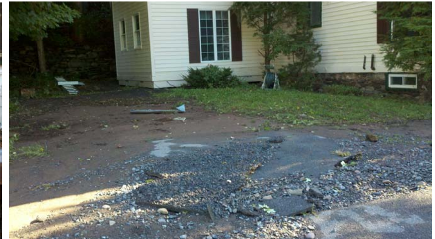
Damage to left driveway
