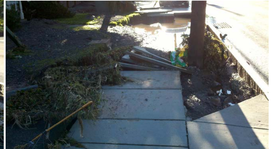
Damage to sidewalk
