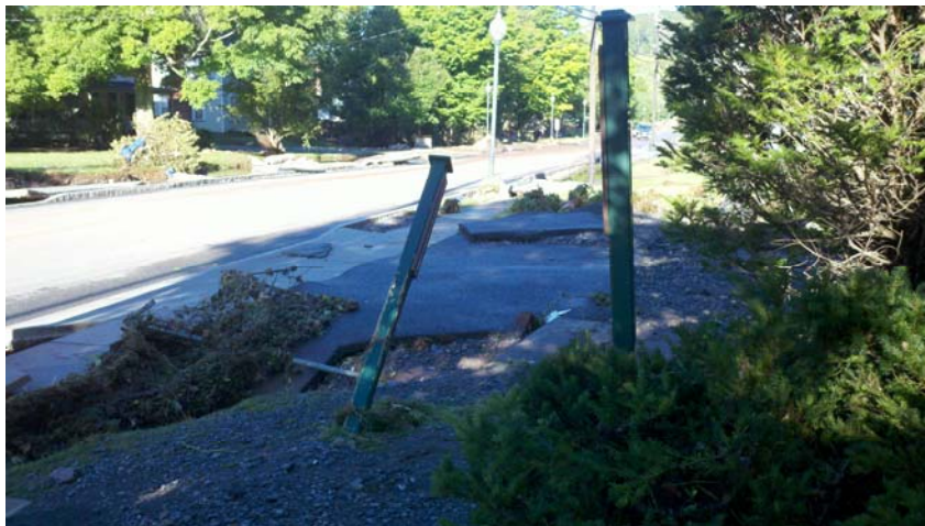
The Law Office of Sean J. Doolan sign was ripped away
